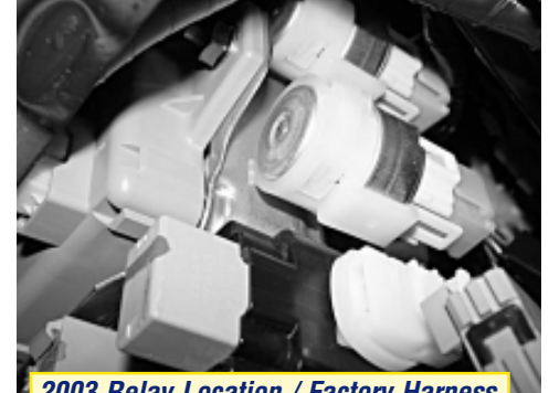
2003 Relay Location / Factory Harness
