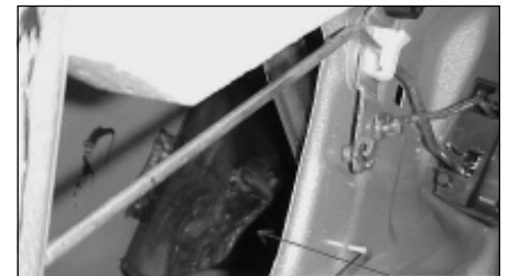
Pad Incorrectly Installed
