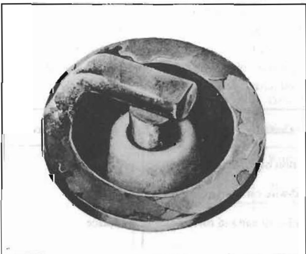
Fig. EE-97 Overheating (I)
