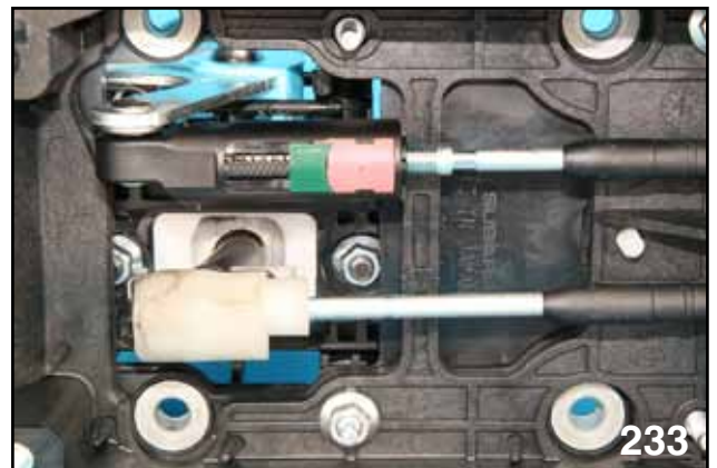
CABLES INSTALLED CLOSE UP
