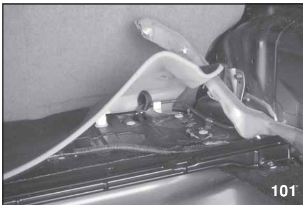
Vent Control Piping
