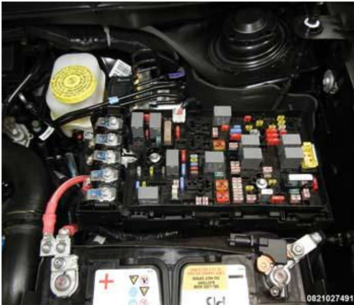
Fig. 1: Power Distribution Center (PDC) Courtesy of CHRYSLER GROUP, LLC
