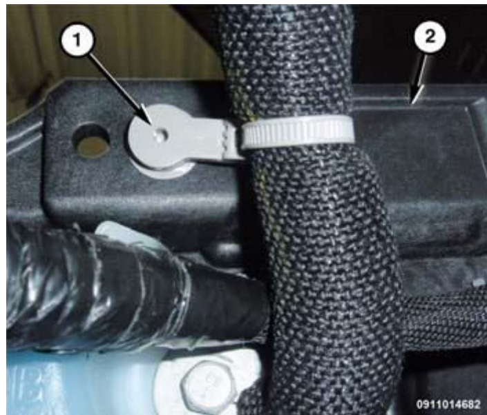
Fig. 32: Battery Tray & Engine Wire Harness Retainer Courtesy of CHRYSLER GROUP, LLC
